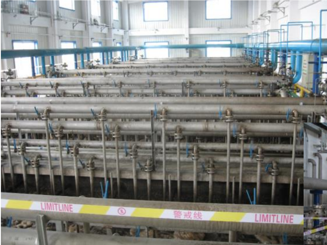
• MBR tanks (7 tanks) in a building: protection from cold weather
